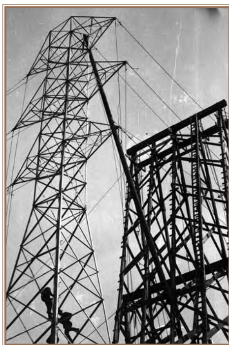
Hetch Hetchy power transmission towers 1924
